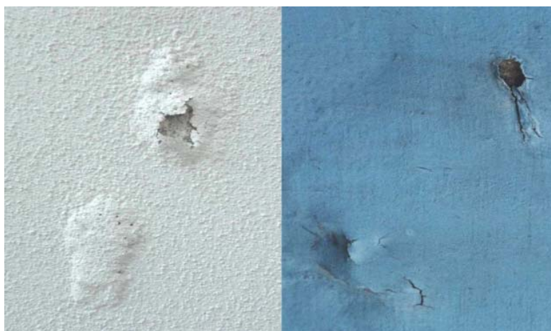
Figure 1: Inadequate permeability to water results in damage to facades.
